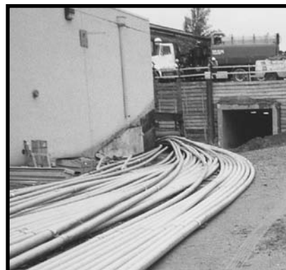
Bore-Gard is flexible enough to be pulled around a building.
