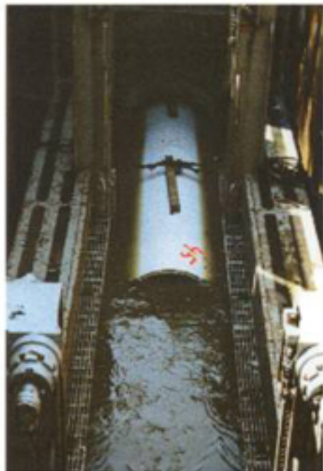
The sewer flows continue uninterrupted at 20 to 80 percent flow capacity during the sliplining process.
