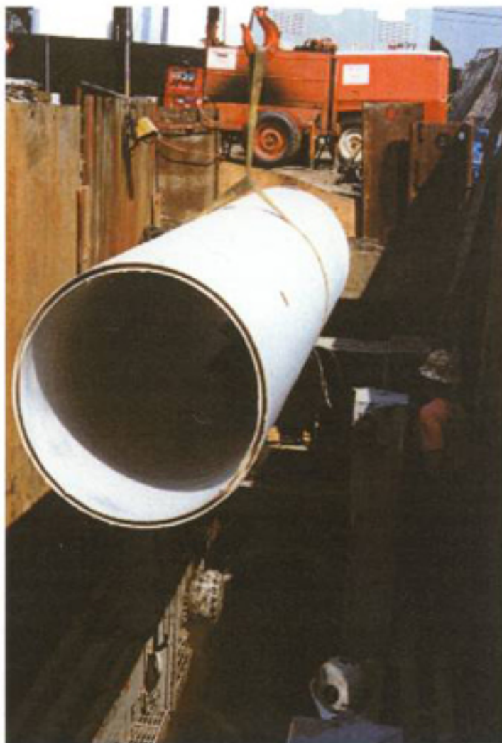
The District 5 Trunk Rehab Project uses 15-ft segments of the 36-in. closed profile-wall PVC sliplining pipe.
