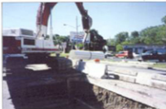
Marra Construction crews lower a 15-ft section of Vylon slipliner into the insertion pit.
