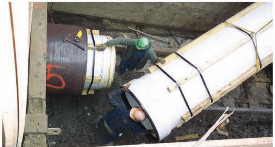
Vylon pipes being connected and inserted into casing pipe for river crossing.
