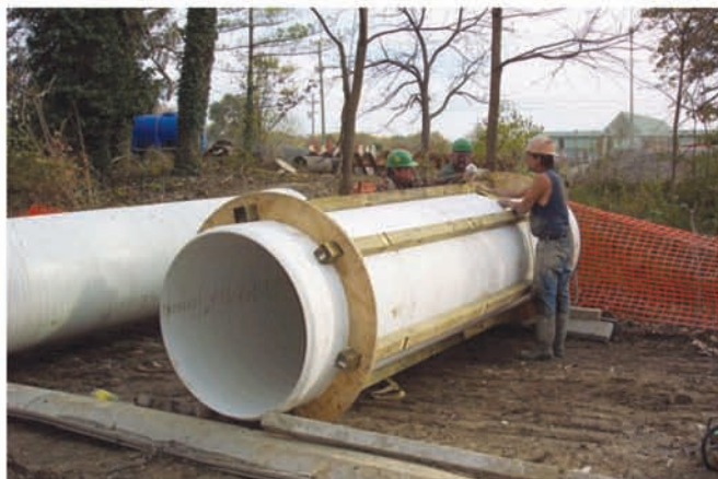
A worker prepares the Vylon pipe for insertion into the steel casing pipe for the river crossing. Six skids were strapped to each Vylon pipe before insertion in the casing pipe per the manufacturer's recommendation. Once in place, the annular space between the Vylon and casing pipe was grouted to prevent flotation.
